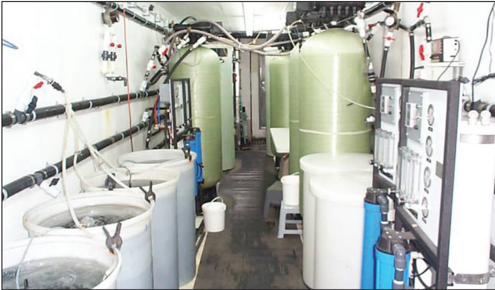
Inside the piloting trailer
