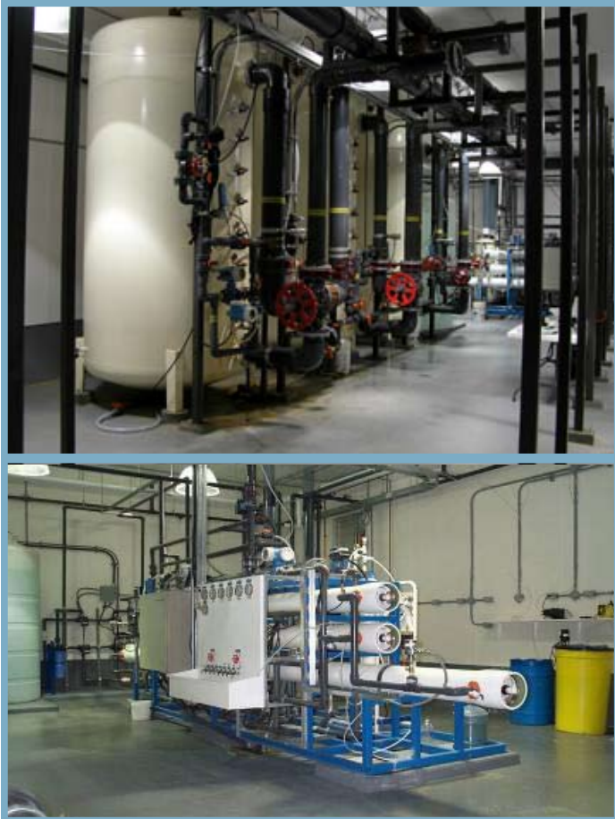
Fig. 6. Upper: full scale biological filters; lower: reverse osmosis treatment unit at the Yellow Quill First Nation water treatment plant.
