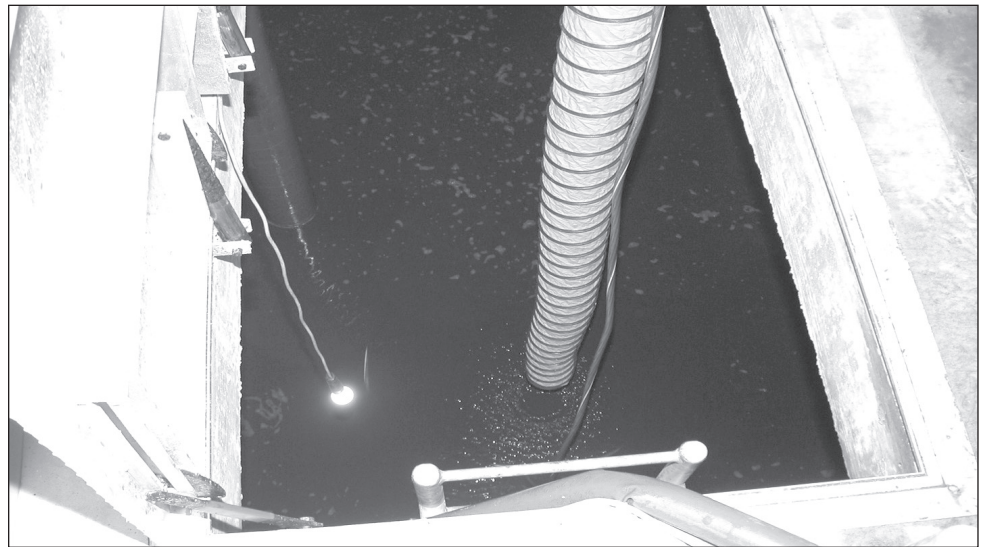
Ooze is all that remained at the bottom of the treated water reservoir from Yellow Quill's old water treatment system. After the IBROM was commissioned you can now drop a quarter to the bottom of the reservoir and years later you can still see that quarter. There is no more ooze.
