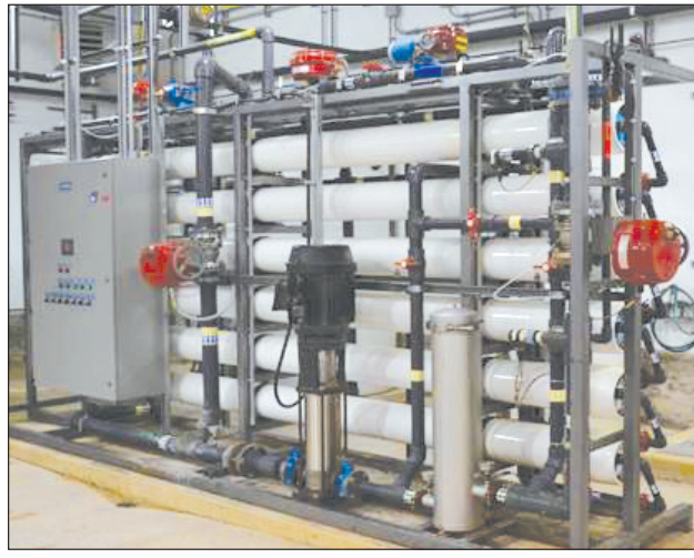
Yellow Quill's RO membrane skid
