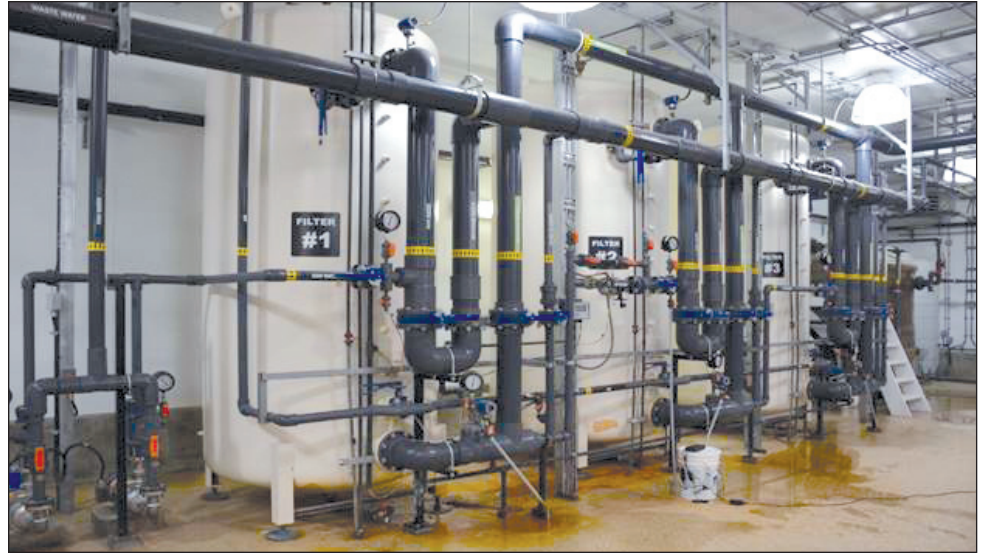
Yellow Quill's biological treatment filters. As described earlier, after the water has been treated in the biological filters it flows to the RO membrane unit. SUBMITTED PHOTO
